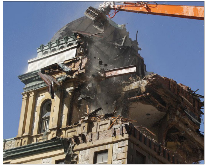
Fig. 13: The demolition of Greystone Asylum and the destruction of its last remaining mansard cupola.
